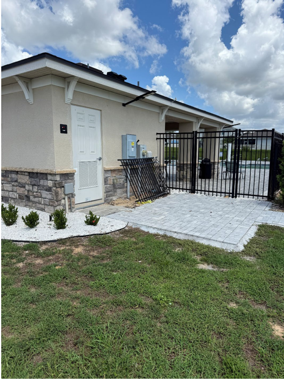
Extra fence pieces left outside of pool area – did not come from pool perimeter fence
